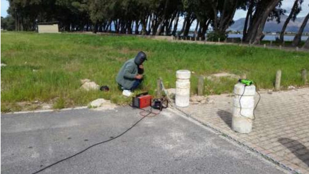
False Bay Nature Reserve staff member Grant Revell attaching (welding) one of the chain barriers to bollards across an access point along the eastern shoreline of Zeekoevlei (Photo: V. Dav 2016)
