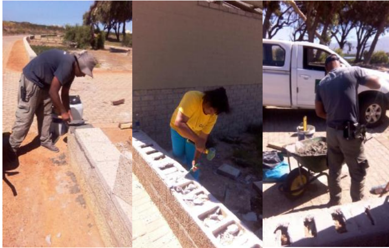
Dylan, Beryl and Henry fixing damage boundary wall (D. Mentor and B. Steers 2017).
