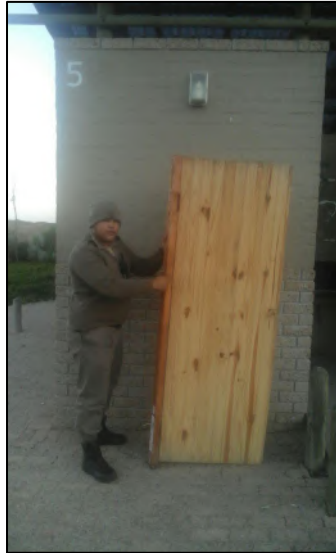
Door found in toilet block no. 5 hanging by its hinges (Photo: Integrity team 2017).
