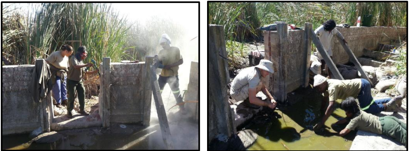
False Bay Nature Reserve staff fixing the Rondevlei weir (Photos: S. Khan 2017).
